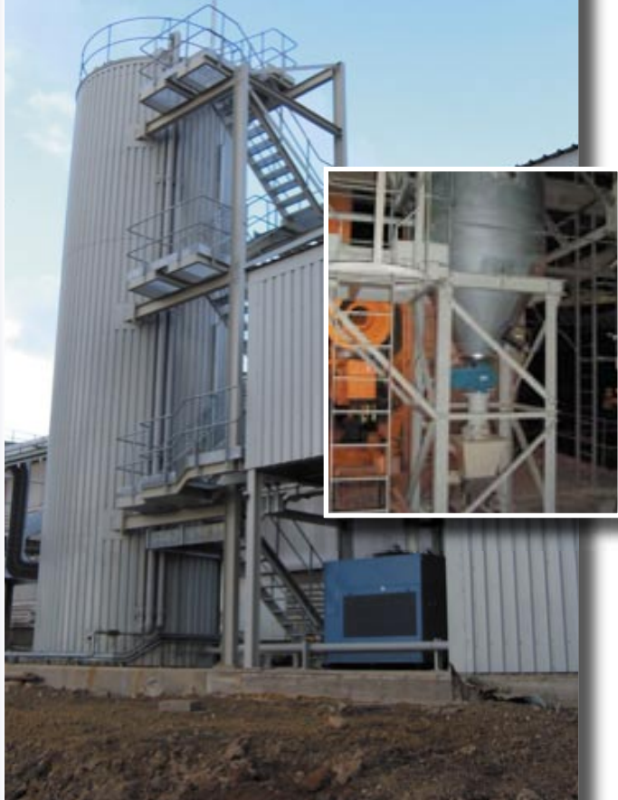
Silo and (inset) loss-in-weight feeder for ferrous sulphate, for Castle Cement by Fairport Engineering.
